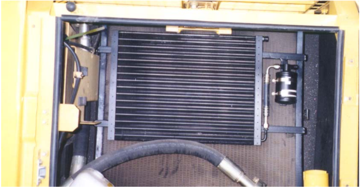
Condenser assembly in place on radiator.
