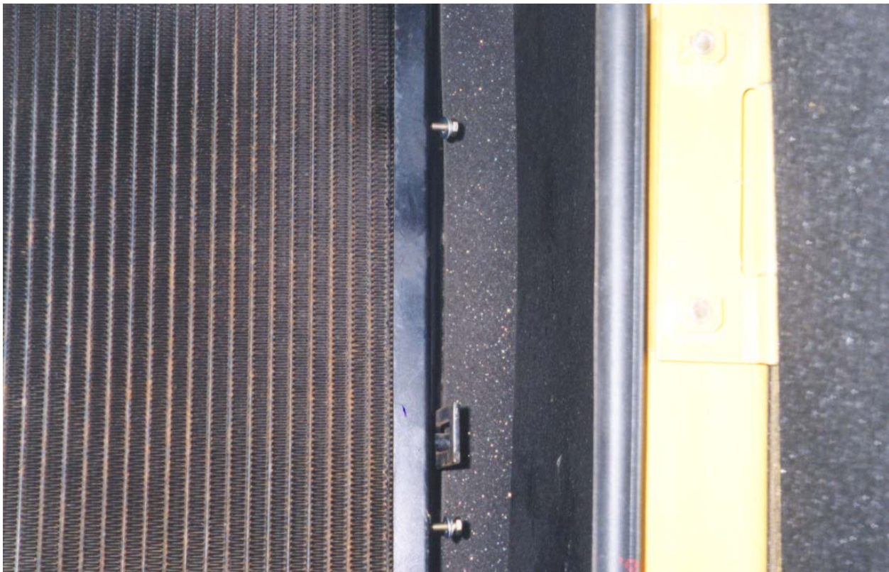
Condenser mounting positions indicated with hardware.
