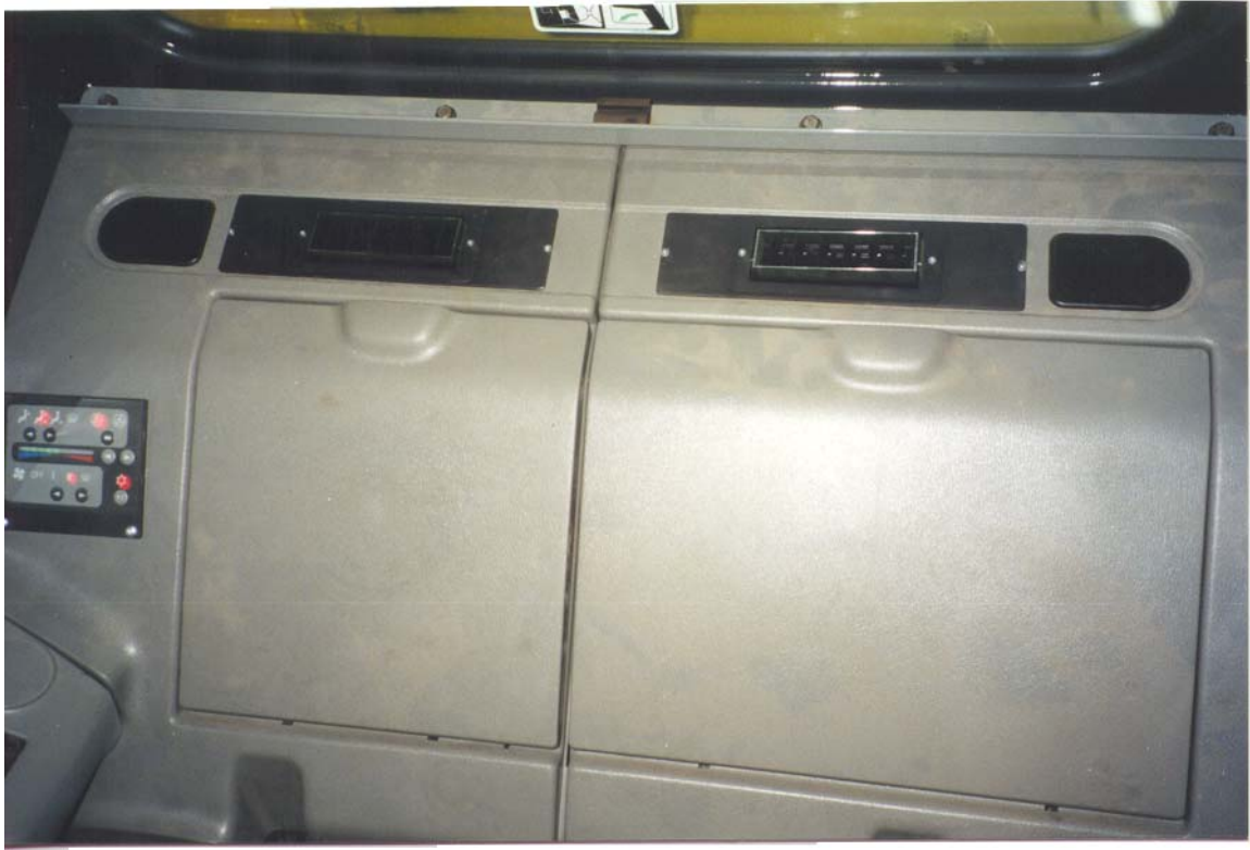
Louvers and controls in place.
